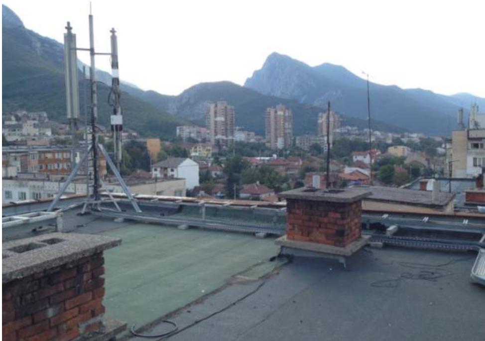
Figure 1: eVolution Networks selected a typical base station for the network and examined the influence of SES on the air-conditioner
